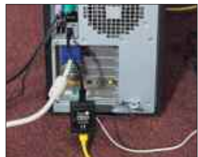
ESP LN installed on the network connection to a PC. Note the black earth lead connection to the chassis of the PC
