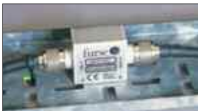
ESP RF 111A11 installed on a coaxial cable running between an antenna and an RF receiver. Note the earth lead (behind the cable tray) attached to the mounting fixture
