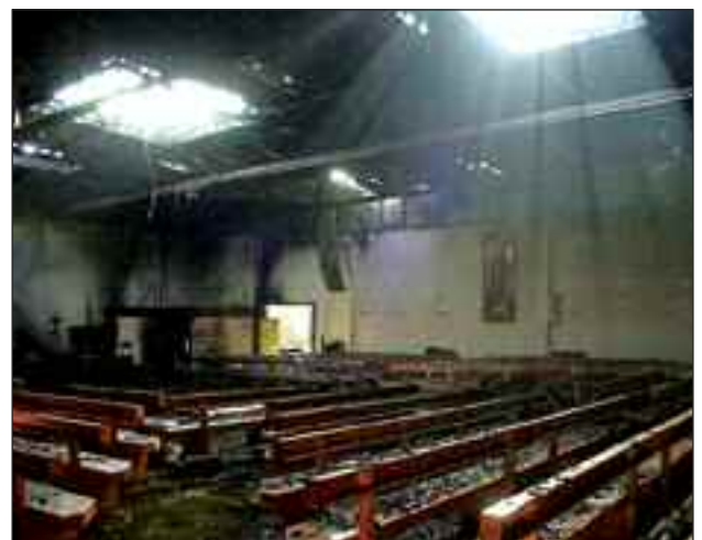
Fires from lightning strikes can cause major damage to structures
