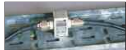
ESP RF 111121 on a coaxial cable running between an antenna and an RF receiver
