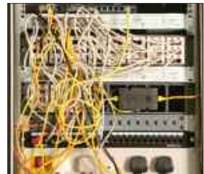
A Furse ESP Cat-5e/Gb protecting a hub from transient overvoltages on a network connection with another building
