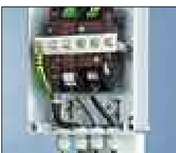
Protectors for the video (ESP CCTV/B, left), camera telemetry (ESP 06E, centre) and the low current mains power (ESP 240-5A, right) inputs to a camera, installed together on a CME 4 mounting and earthing kit. Note that the protectors have been cross bonded to the metalwork of the pole (out of shot)
