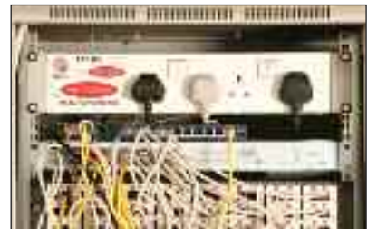
ESP MC installed within a network rack, protecting the externally-fed network switch
