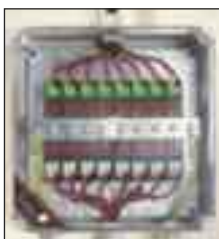
Protectors installed on a combined mounting and earthing kit (CME 8) within a WBX 8 enclosure
