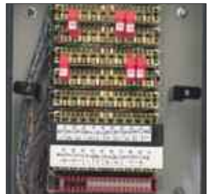
Single line protectors installed on LSA-PLUS disconnection modules, via ESP KE10 earth bars, on all incoming signal and data lines
