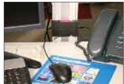
An ESP TN/RJ11-4/6 protecting an external fax line. Note the short earth connection made to the local ring main
