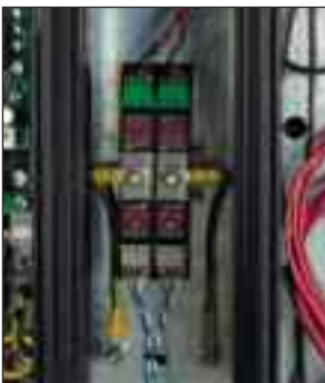
Two ESP 15H protectors mounted in a control cabinet and earthed via the cabinet's earthed chassis
